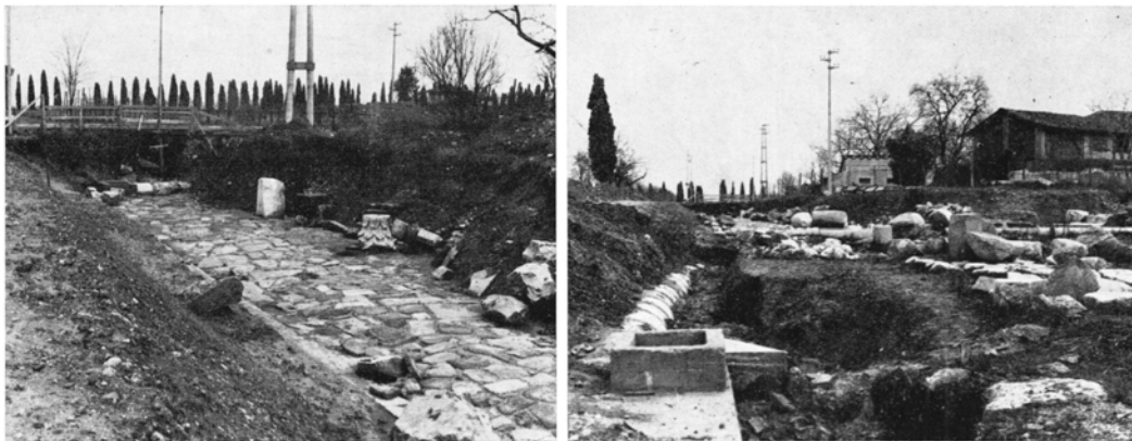
Illustration 3 | left: the Decumano discovered; right: the sewage system under construction along the Decumano.
