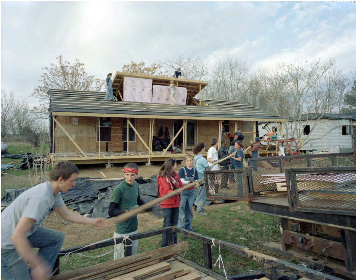
Figure 5 | The students learn by building the house from the foundations to the exterior finishing.
